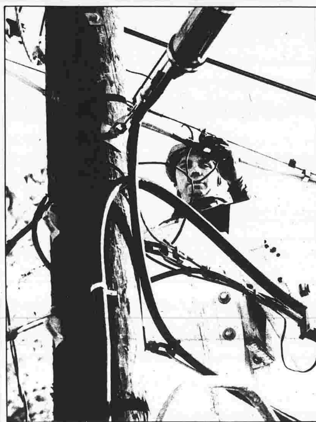
Steve Pryor, a lineman for Cox Cable Greater Hartford, repairs lines on Spruce Street Sunday. Last week's snowstorm knocked out service to a number of cable television subscribers in the Manchester area, but all were said likely to be back on line today.
